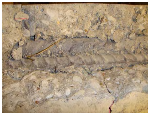
Figure 5.13 Enamel coating remained on steel rebar.
