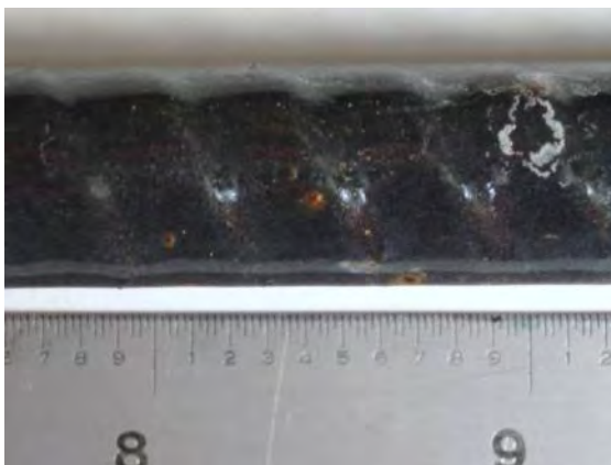
(a) “Minor” signs of corrosion
