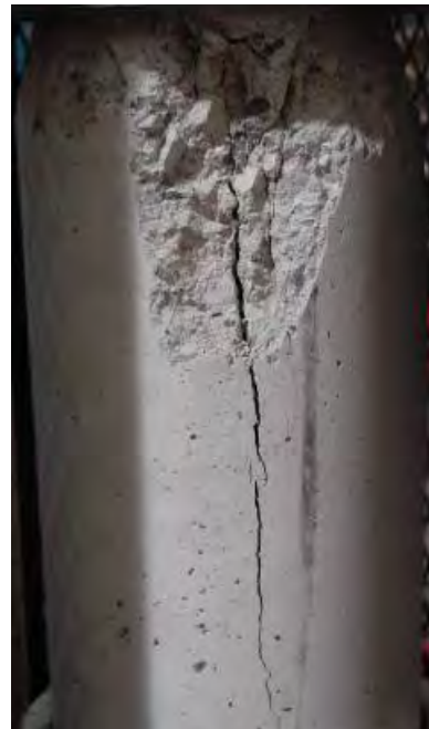
(b) Failure mode
