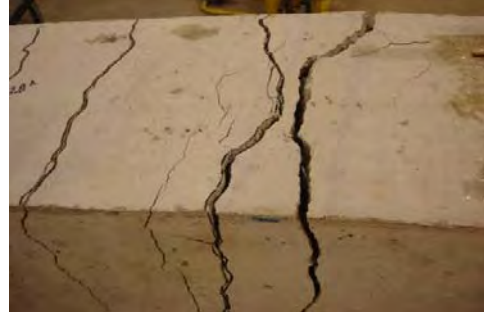
(c) Cracks at failure
