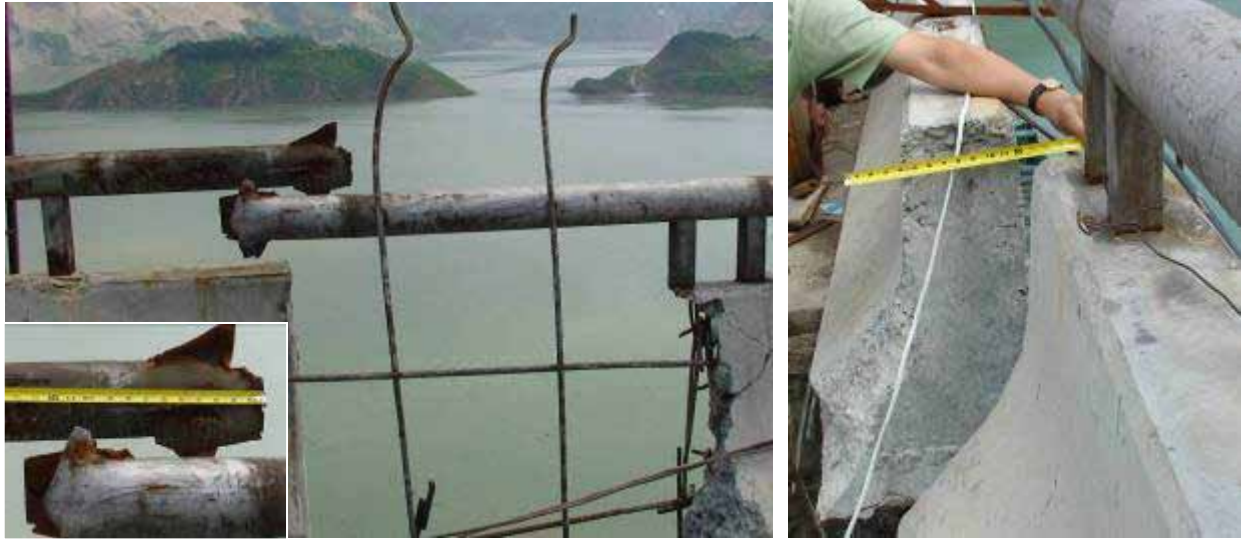
Figure 56. Photo. Longitudinal and Transverse Offset of Bridge Deck.
