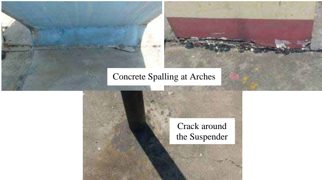
Figure 37. Photo. Concrete Spalling and Cracks on Bridge Deck.
