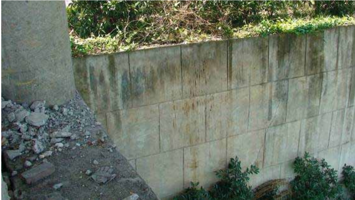
Figure 44. Photo. Crack on Retaining Wall Underneath the Northwest Approach.
