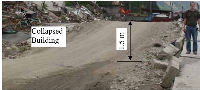
Figure 6. Photo. Surface Rupture Along the Old Highway Near a Collapsed Building.
