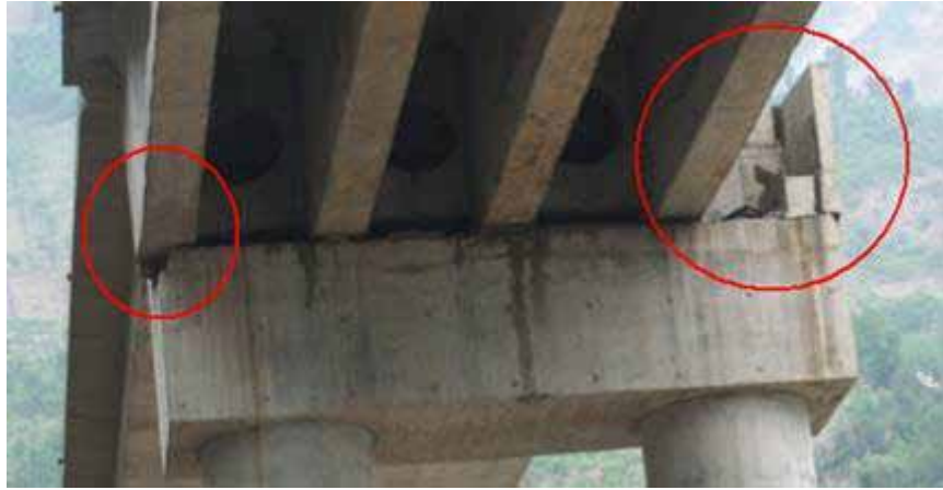
Figure 66. Photo. Damage at Bent 9.
