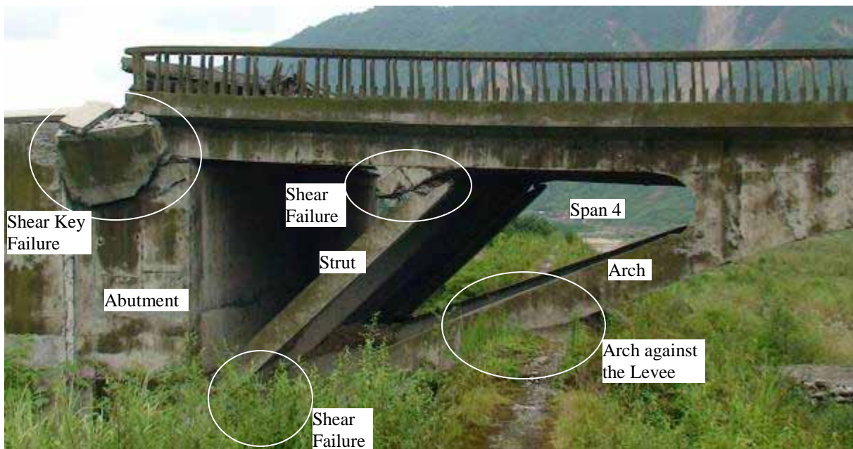
Figure 19. Photo. Damage in Easternmost Span.
