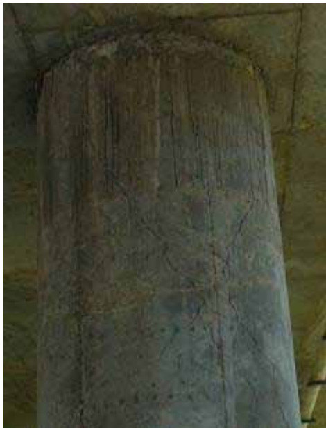
Figure 43. Photo. Shear Crack at East Column of Bent 5 of the Northwest Approach.
