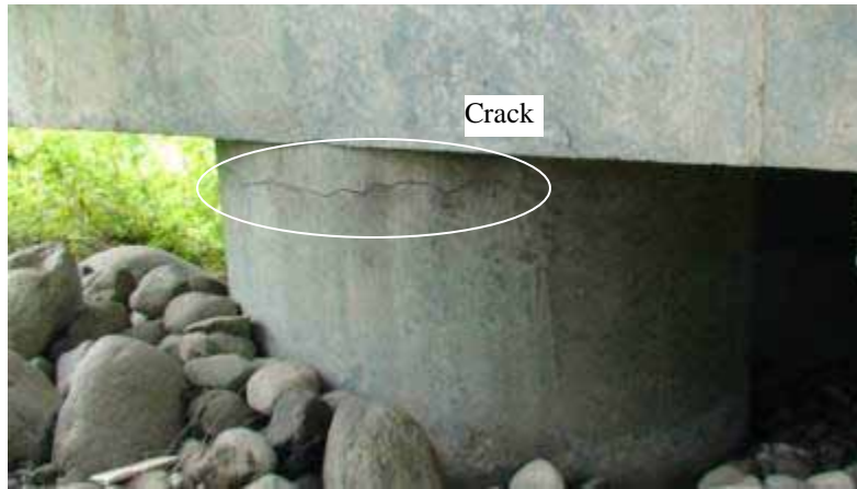
Figure 22. Photo. Flexural Crack on Pile Shaft at Bent 4.
