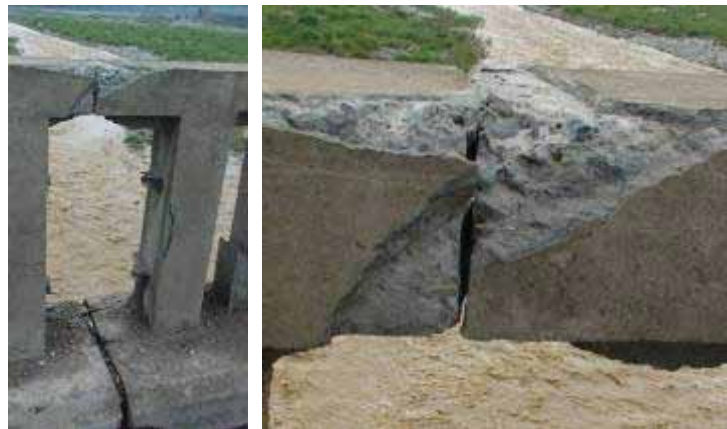
Figure 14. Photo. Pounding Damage at Railing Joints.
