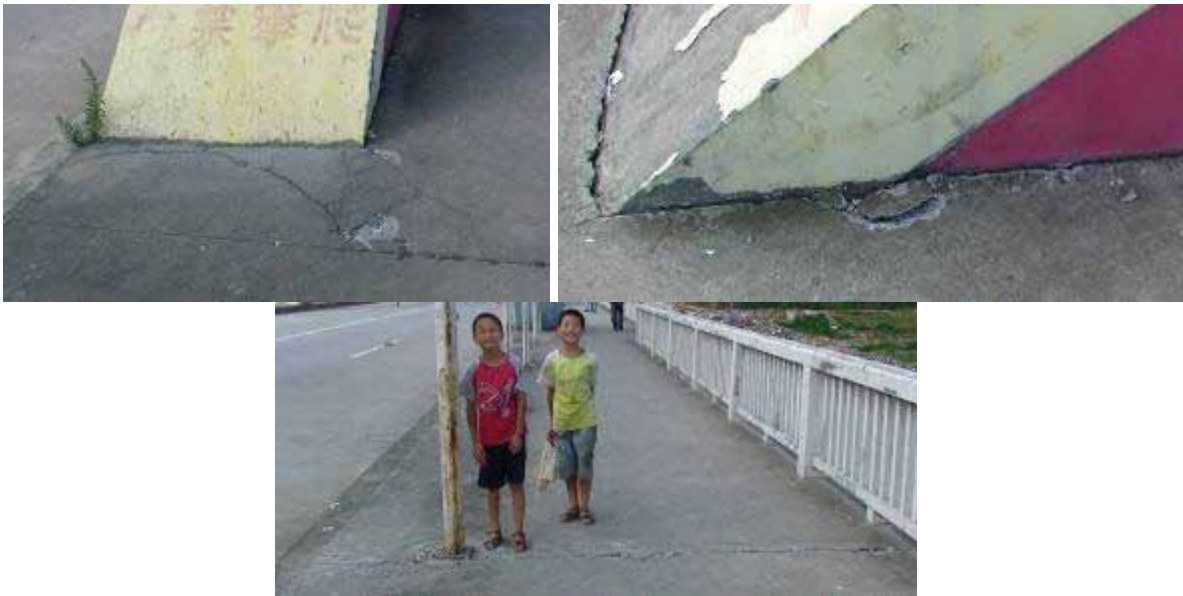
Figure 27. Photo. Damage in Bridge Deck Around Arch and Suspender.
