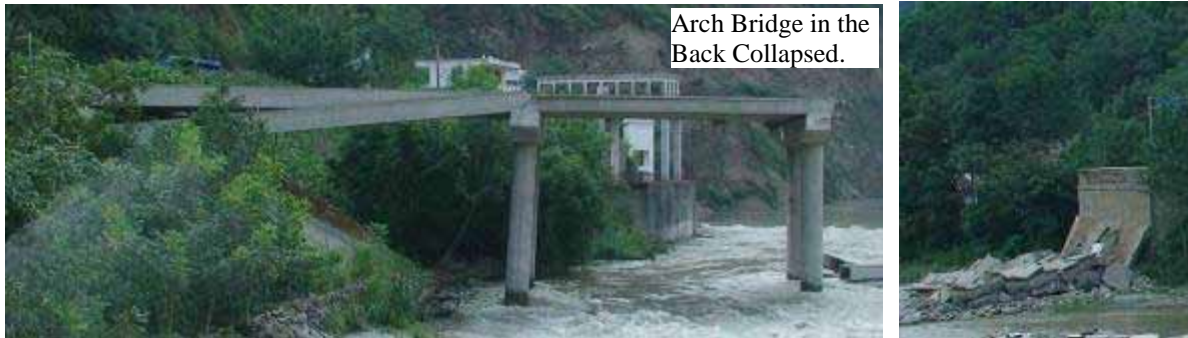
Figure 46. Photo. Collapse of the Old Three-Arch Bridge.
