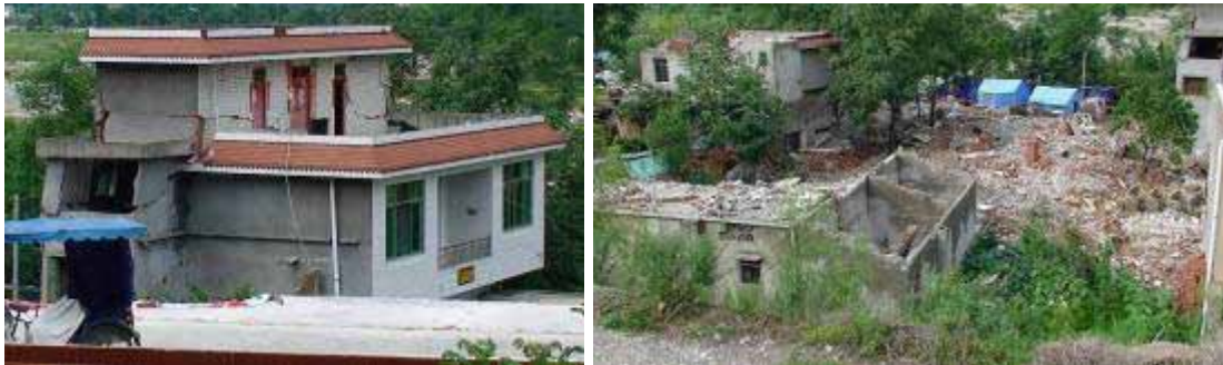
Figure 33. Photo. Building Damage in Nearby Town.
