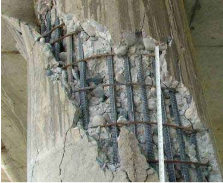
Figure 42. Photo. Shear Failure at West Column of Bent 5 of the Northwest Approach.
