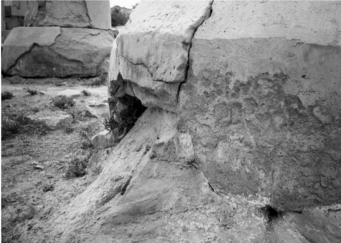
Figure 2. Photograph of deteriorated stone foundation at the Karnak Temple complex.
