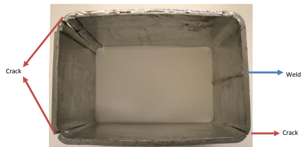
Figure 1. Cracks seen in the galvanized ultra high strength hollow structural steel (HSS) tubing.
