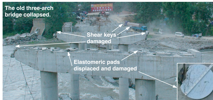
FIGURE 3 Collapse of old arch bridge and 10-span bridge.
