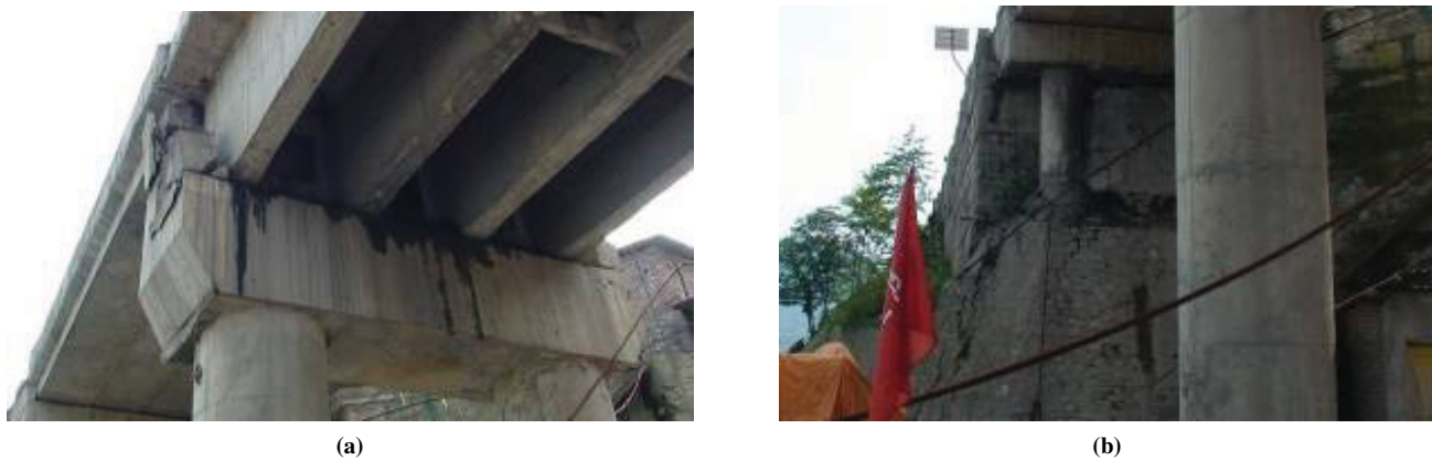
FIGURE 11 Damage to shear key and embankment of the overpass.
