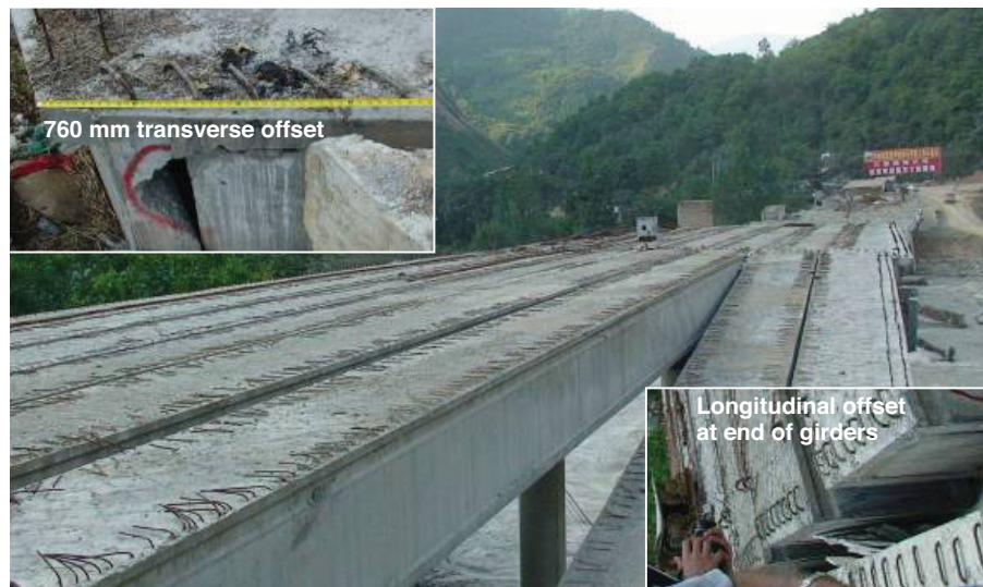
FIGURE 4 Damage to 10-span bridge under construction.
