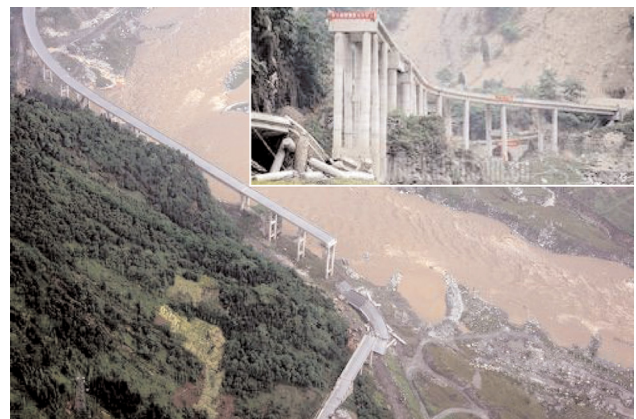
FIGURE 14 Postearthquake damage. (Source: CNS.)
