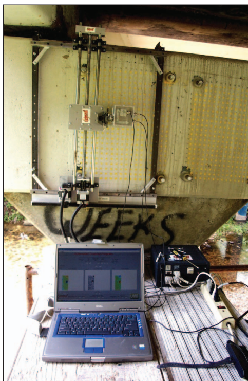
Fig. 2. The dual-polarized microwave reflectometer attached to a scanning platform while inspecting a CFRP patch bonded to the bent of a bridge.
