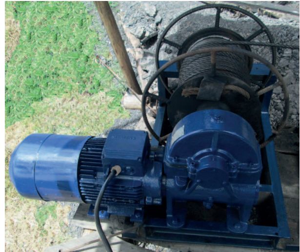
Figure 15. Electric winch. Cochinillos mine location.
