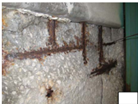
Fig. 2 Cracking and spalling at bridge deck panel joints.
