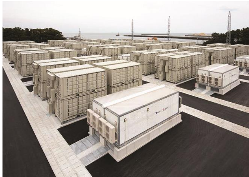
Figure 1.10. Stationary battery units. Courtesy: Mitsubishi Electric [30]
