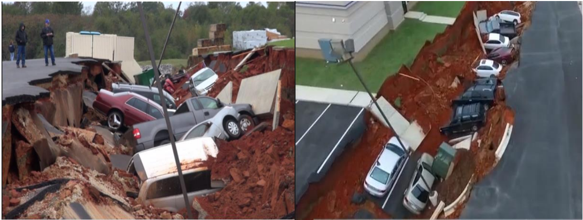
Figure 2.2. Sinkhole Collapse at Parking Lot in Meridian, Mississippi (CNN, 2015)
