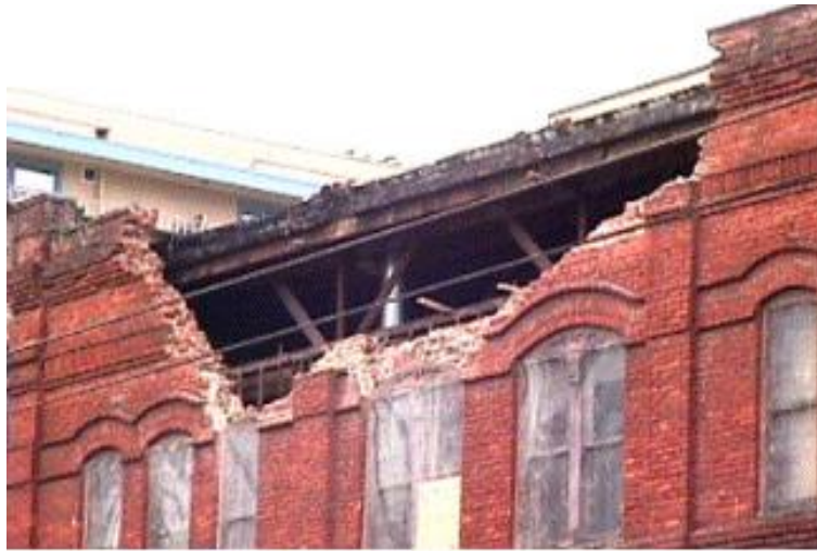
Figure 2.2. Failure of unreinforced wall due to out-of-plane seismic forces [Nisqually Earthquake, 28 February 2001].
