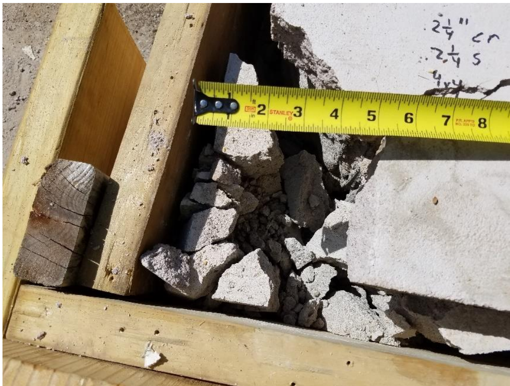
Figure 5.5. Breakage of Substrate, Test 7 8/18/16
