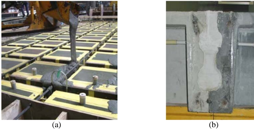
Figure 2-11 Model ribbed slab for validation tests. a) Casting - b) Cold joint (Toutlemonde et al., 2007)
