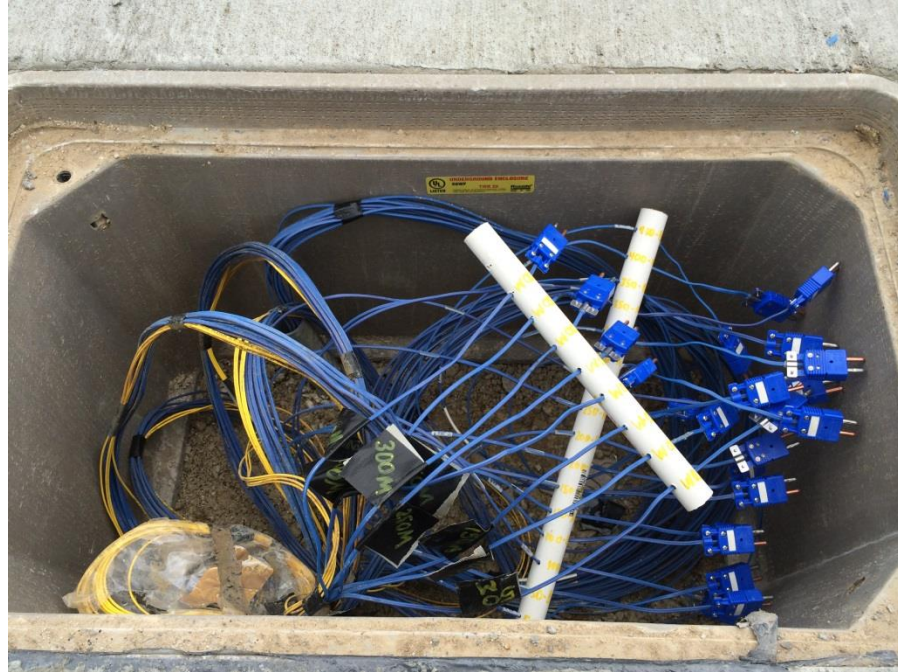
Figure 1.7 Photograph of thermocouple wire enclosed in concrete electrical box.
