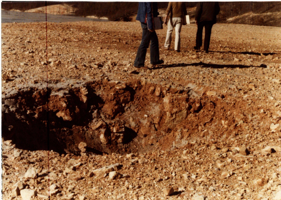
10. Crater-like feature on surface of spoil from spillway excavation. Apparently a result of boulder in spoil sinking into soft tailings underneath. Located about half of the way between left end of dam and spillway.
