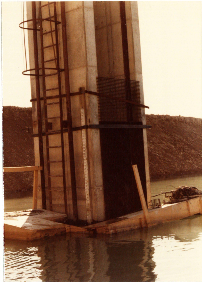
9. Inlet tower for decant line.
