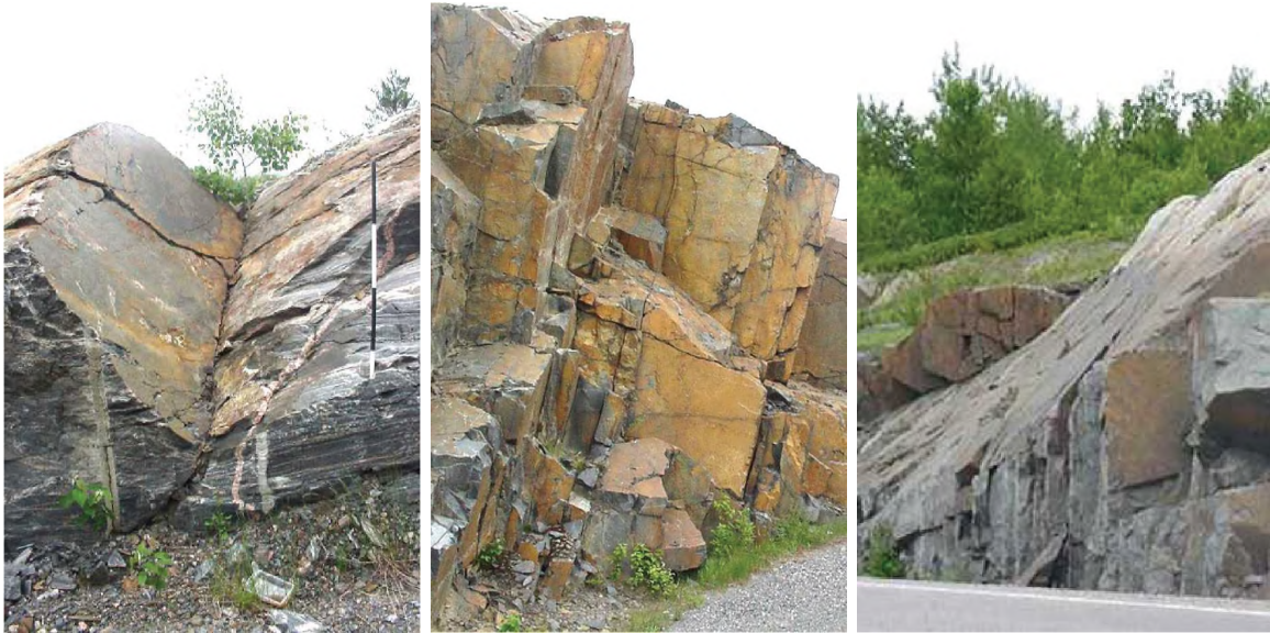
Fig. 1 Example of (a) wedge; (b) toppling; (c) planar failures along road cuts.
