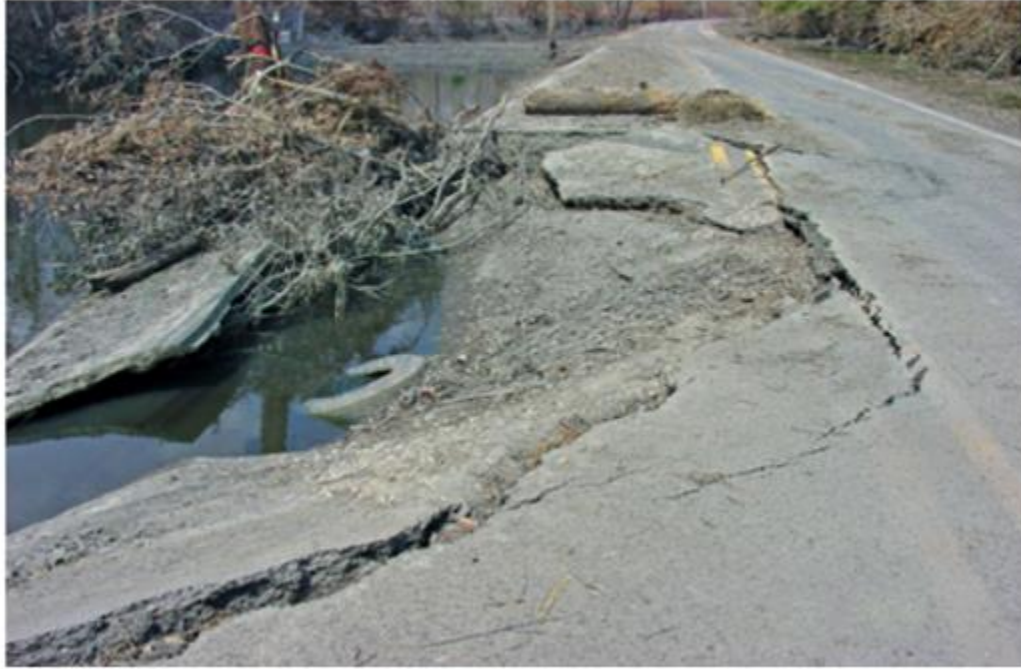
Figure 1.1. Effect of Hurricane Katrina on the roadways of New Orleans, Louisiana. (Image from Louisiana Department of Transportation and Development)
