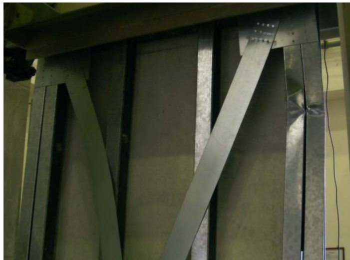
Figure 8 Local buckling of chord studs
