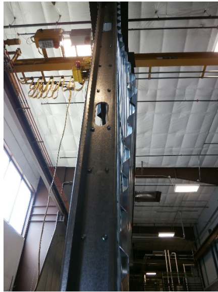
Figure 11 - SW sheathing connection failure
