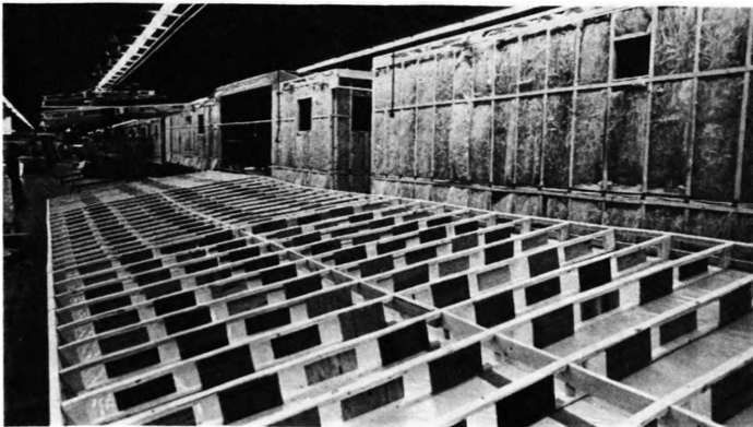
Fig. 13. Main Assembly Line (End-by-End Type): Roof Section Installation (Richardson Homes Corp., Elkhart, Ind.)
