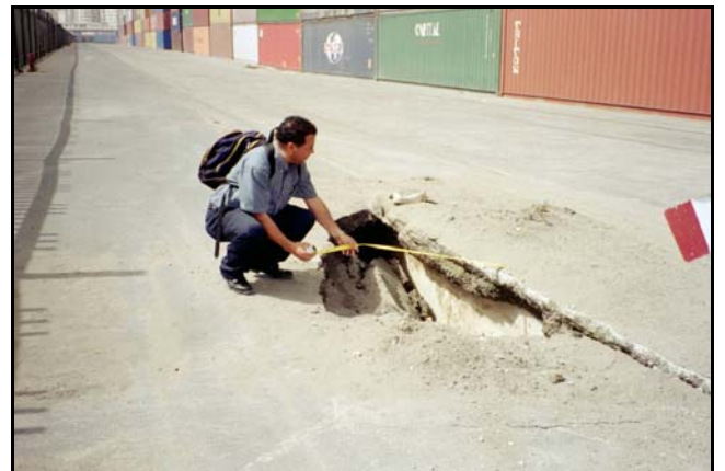
Fig. 21. Cavity caused by loss of soil support due to liquefaction at the Port of Algiers
