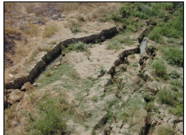
Fig. 13. Close-up view of tension cracks caused by lateral spreading of the riverbank
