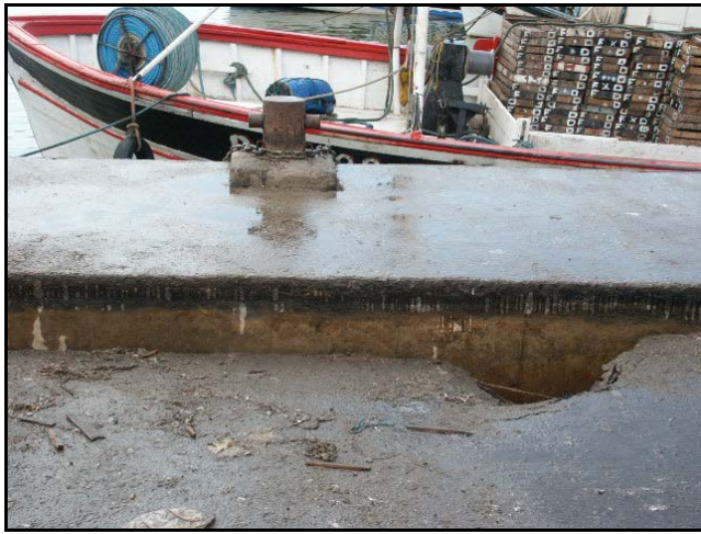
Fig. 22. Settlement ( >0.3 m) behind pier in the harbor of Zemmouri El-Bahri
