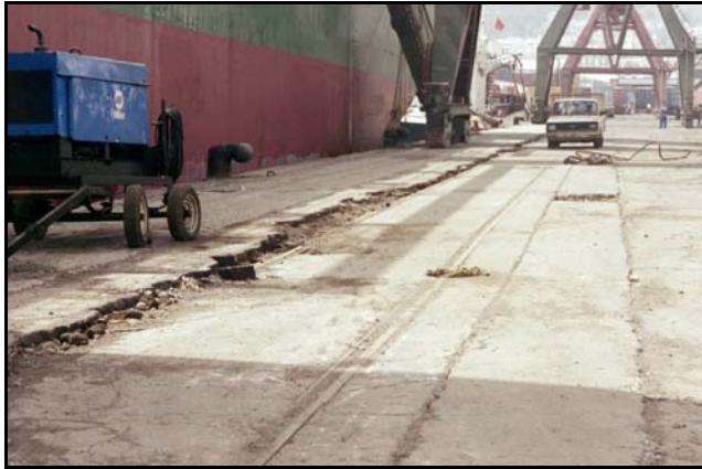
Fig. 18. Differential settlement between quay wall and down-dropped backland, Port of Algiers
