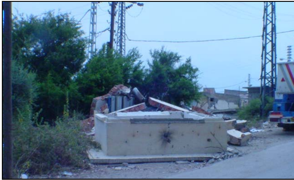
Fig. 7. Concrete cap thrown from its original location
