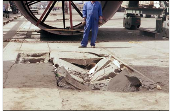
Fig. 20. Loss of ground support under concrete pavement at the Port of Algiers
