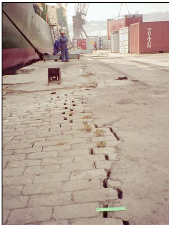
Fig. 19. Tension cracks longitudinal to the quay wall indicating lateral wall movement at the Port of Algiers
