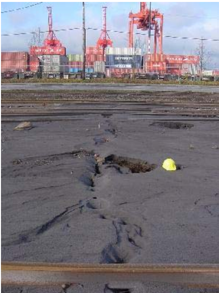
Fig. 20. Sand ejected from a ground fissure crossing railroad tracks at the Port of Seattle. The opening was found to run through the road into the port facilities seen in the background. All ground photos were georeferenced using GPS receivers ( N47.58487^{\circ} W122.33980^{\circ} ), (from Bray, et al, 2001).
