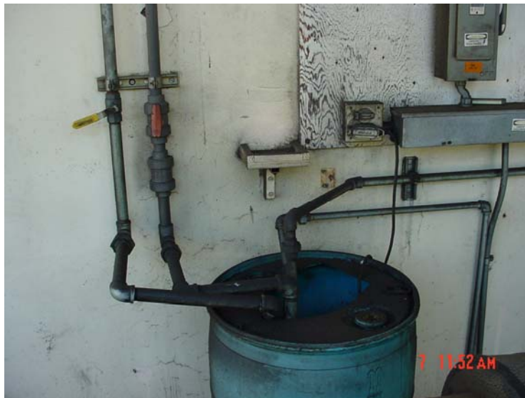
Figure 12 Drum for collecting condensation
