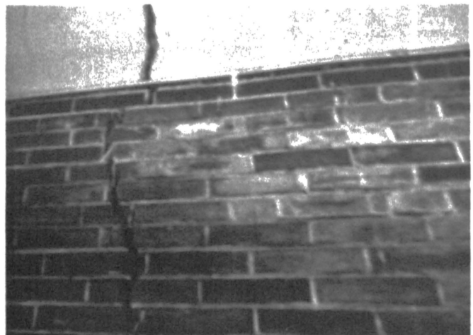
Figure 3. Cracks in classroom walls and ceilings.
