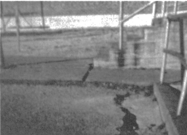
Figure 5. Crack in playground.
