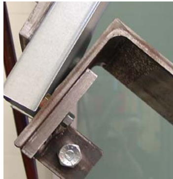
Figure 9. Deformed Deck Around Contour of Weld
