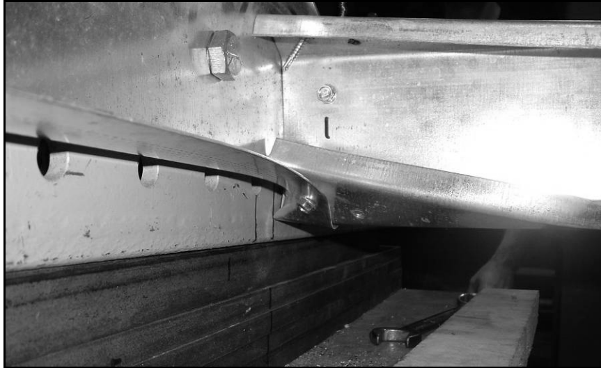
Figure 8: Photograph of Track Punch-Through Failure
