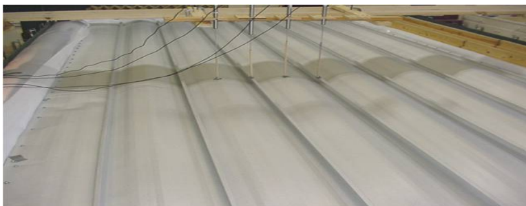
Fig 10. Uniform Static Pressure Tests- ASTM E-1592. Houston Vertical Legs Roofs – During Loading.
