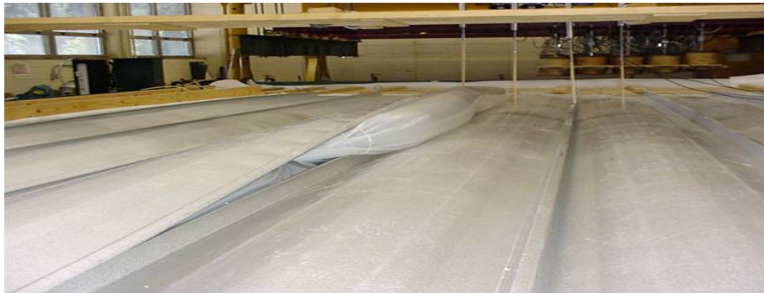
Fig 11. Uniform Static Pressure Tests- ASTM E-1592. Houston Vertical Legs Roofs – After Failure of Seamline.
