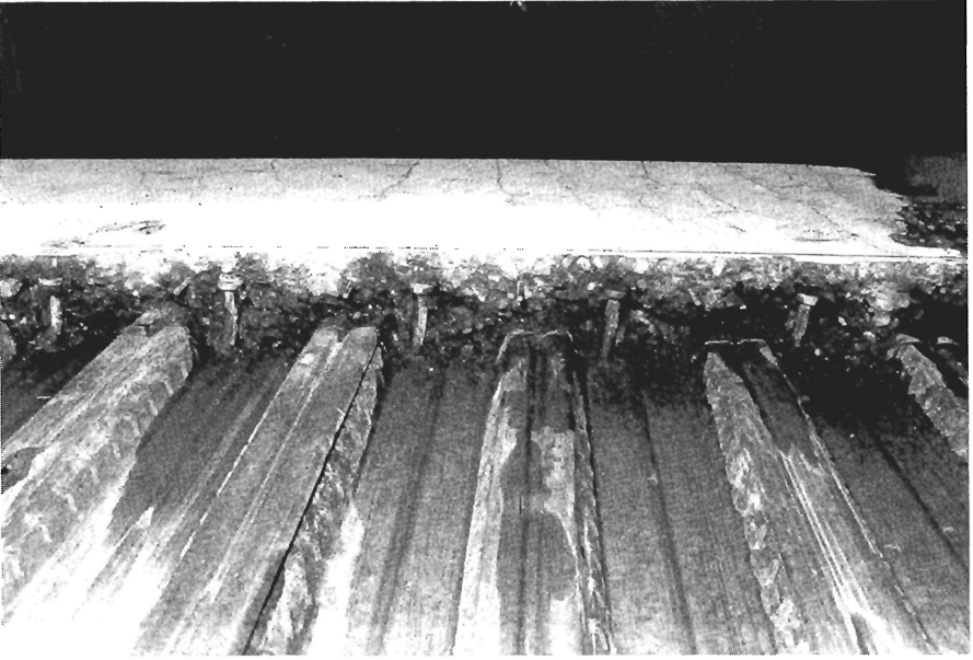
Fig.7 Failure in shear connection
