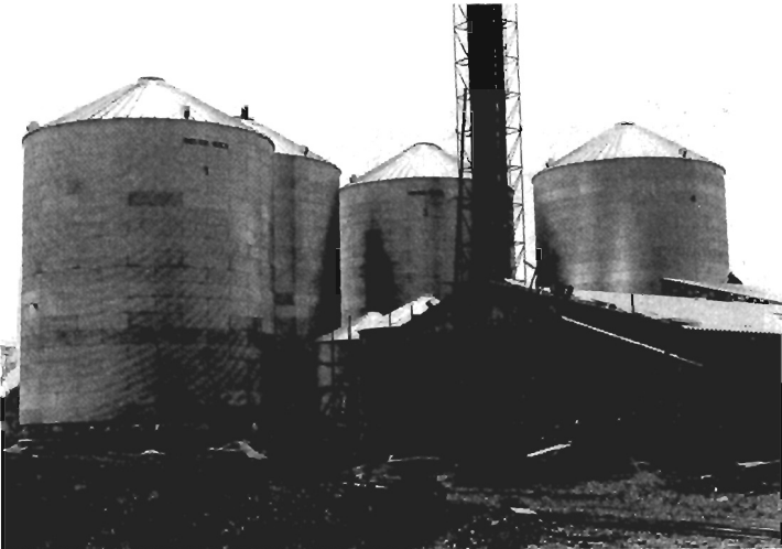
Figure 11. Erection of Bins by Raising Cylinder and Roof and Adding Sheets at Ground Level
