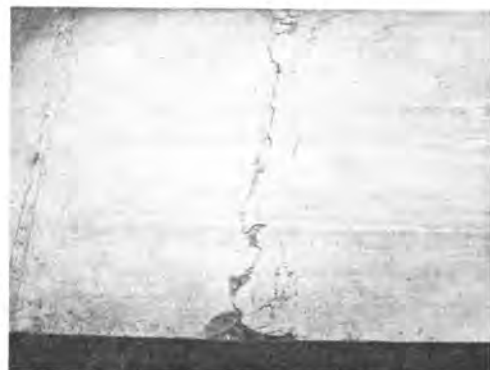
Fig. 8. Crushing concrete failure of beam element.
