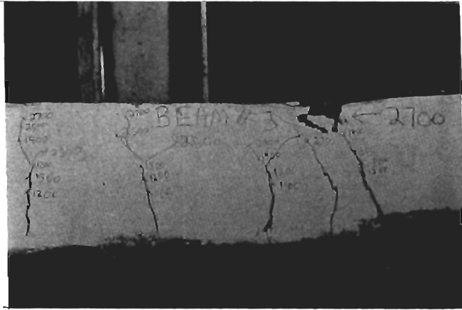
Fig. 4b: Beam No. B-6 after Failure (Tension Failure)
