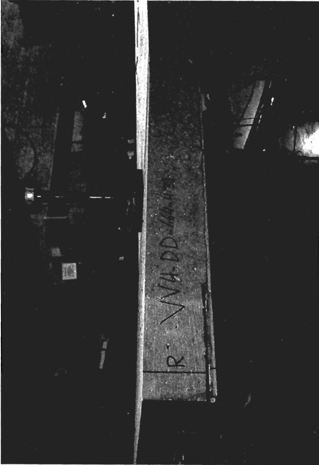
Figure 7. Typical Shear-bond Failure, Showing Failure Crack.
