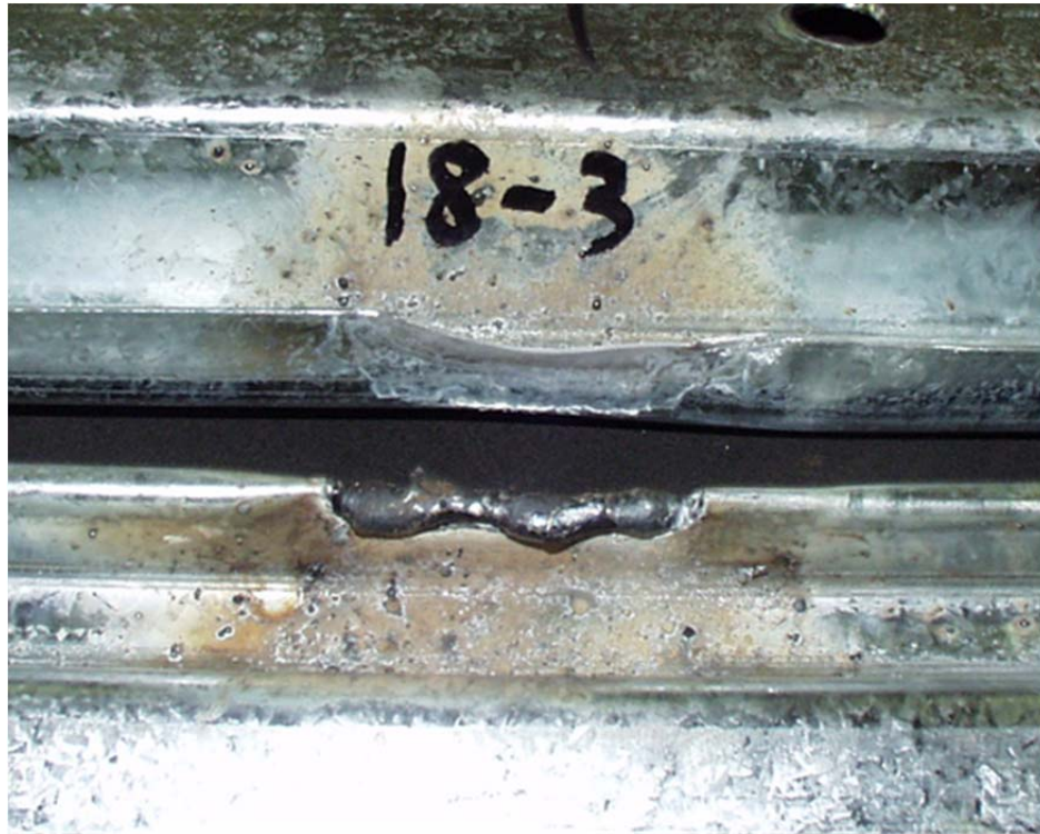
Figure 4 Typical top seam weld failure (shearing of male leg parallel to weldment)
