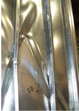
Figure 7: Distortion of interior studs
