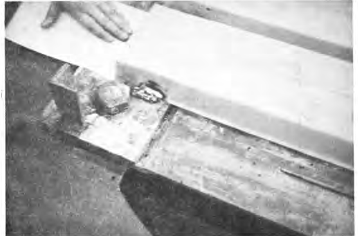
Fig. 9. Tearing of Sheet Around Weld and Displacement
