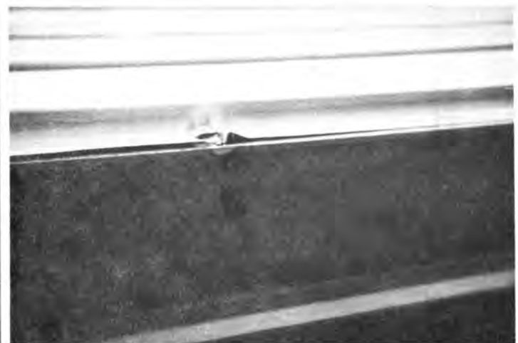
Fig. 10 Sheet Tearing and Displacement
