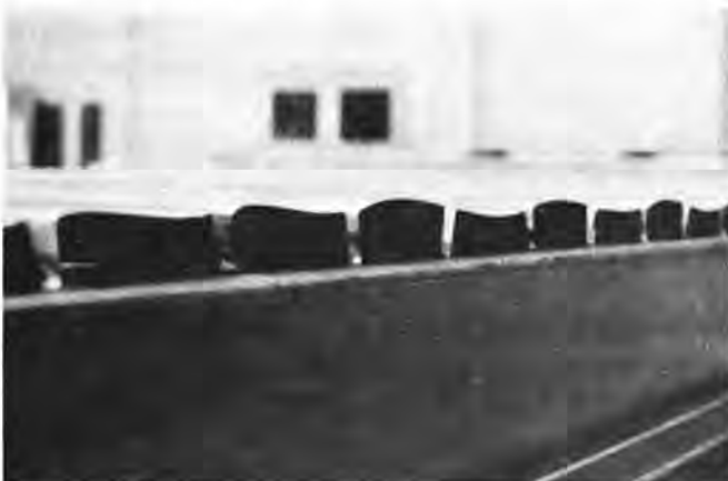
Fig. 17. Warping of Steel Deck at Ends
