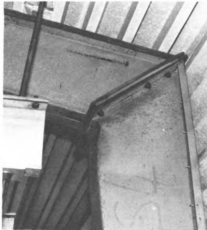
Fig 11 Eaves after failure.
