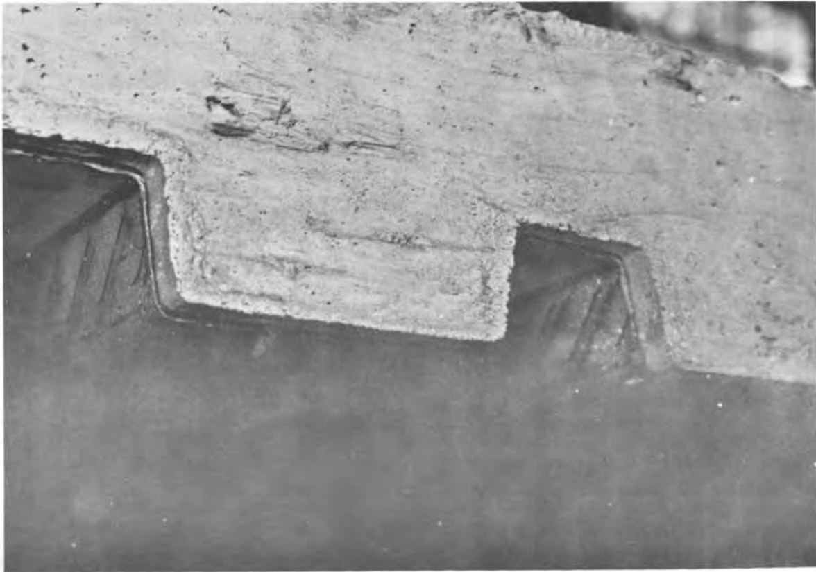
Fig. 8. Photograph of end-slip after failure of a one-way slab element.
