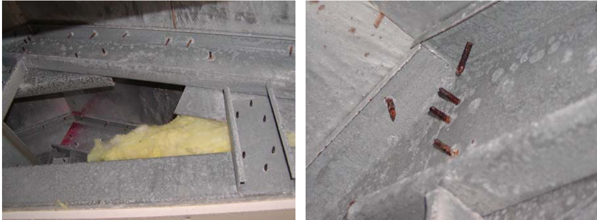
Figure 7.25: Vented attic framing at MCBH Coastal after 16 months.
