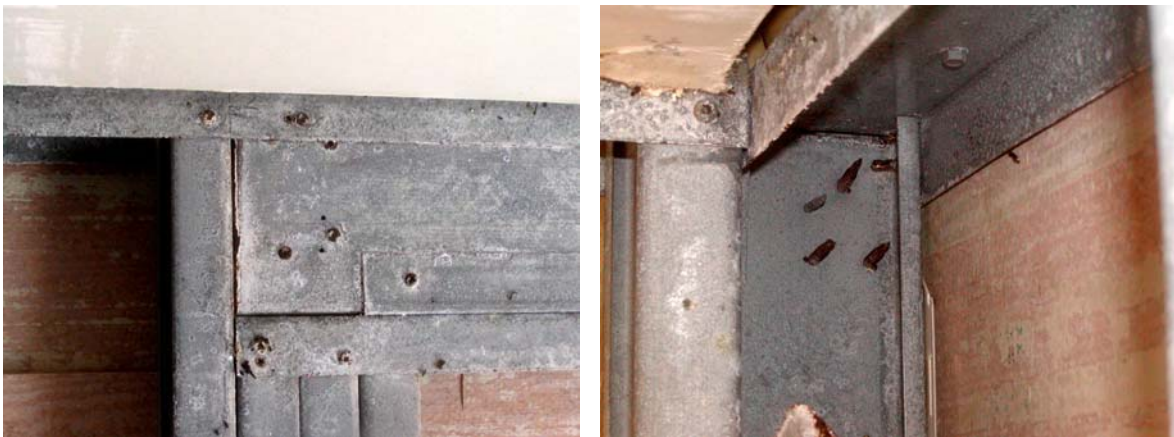
Figure 7.20: Wall framing with lap siding without vapor barrier, MCBH Coastal after 21 months.
