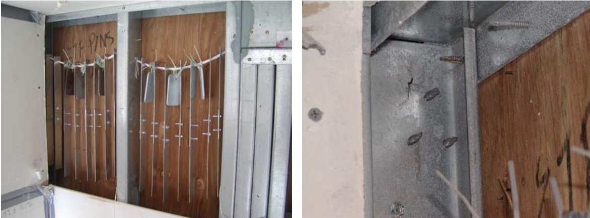
Figure 7.8: Wall framing with plywood sheathing at MCBH Inland after 28 months.
