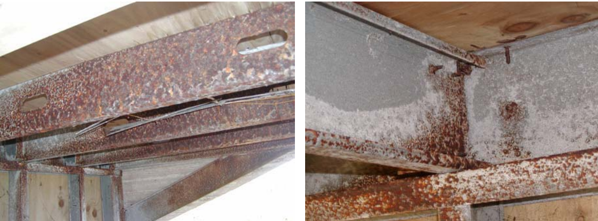
Figure 7.38: Crawl space exposed floor joists, MCBH Coastal after 28 months.
