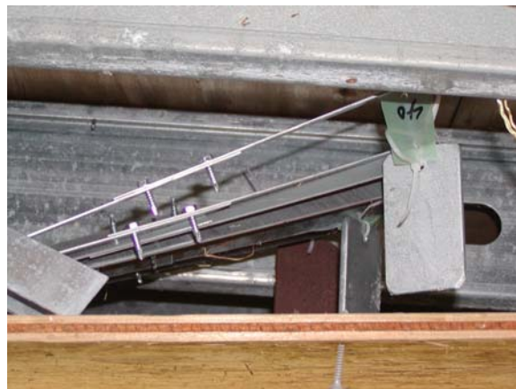
Figure 7.15: Floor joist with plywood sheathing after 28 months exposure.
