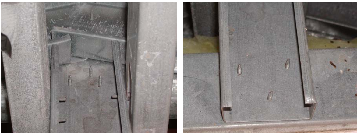
Figure 7.9: Vented attic framing at MCBH Inland after 28 months exposure.
