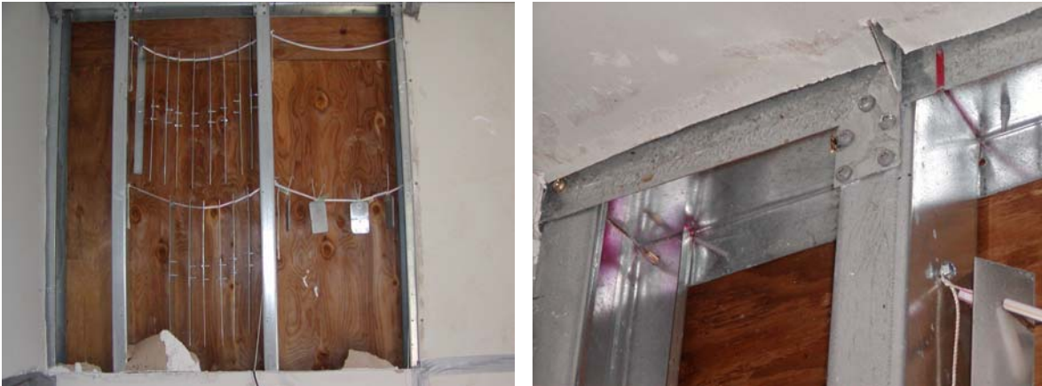
Figure 7.1: Interior wall framing and fasteners at Iroquois Coastal site after 20 months exposure
