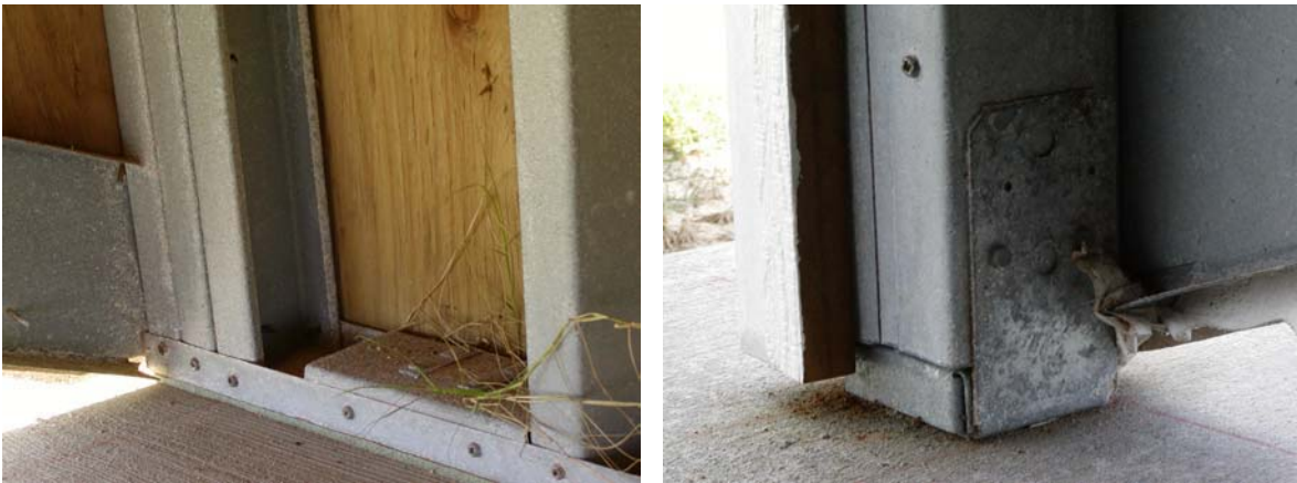
Figure 7.28: Crawl space cripple wall and post, MCBH Coastal after 5 months.
