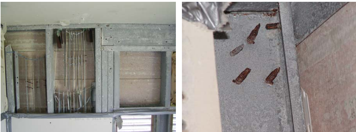
Figure 7.21: Wall framing with lap siding without vapor barrier, MCBH Coastal after 28 months.
