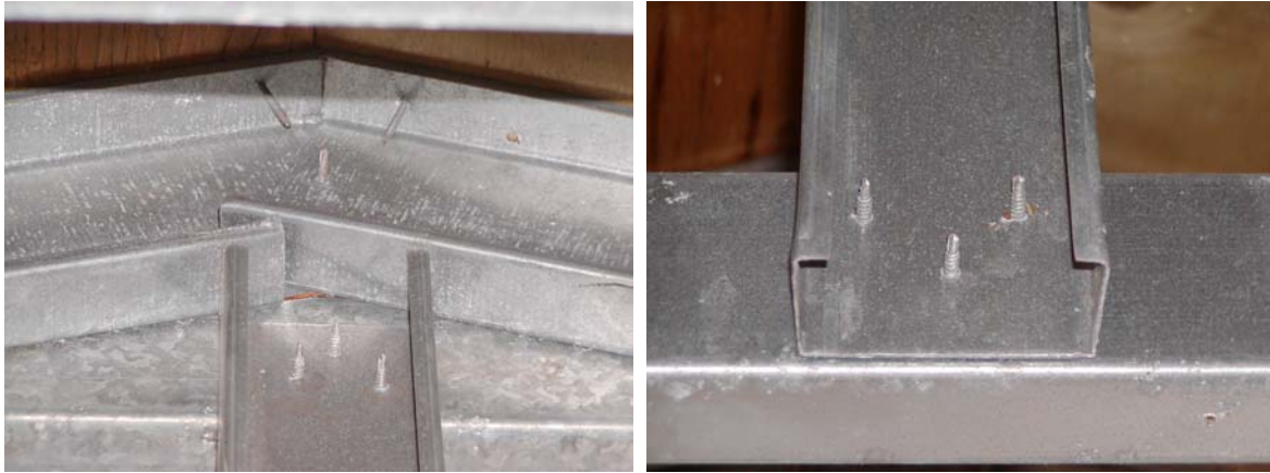
Figure 7.3: Attic framing at Wheeler site after 20 months exposure.
