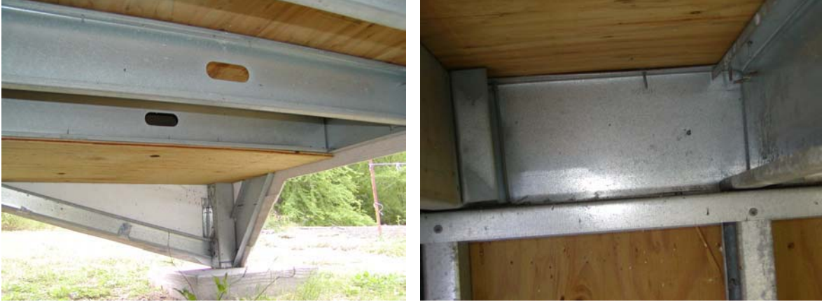
Figure 7.13: Crawl space floor joists at MCBH Inland after 16 months exposure.
