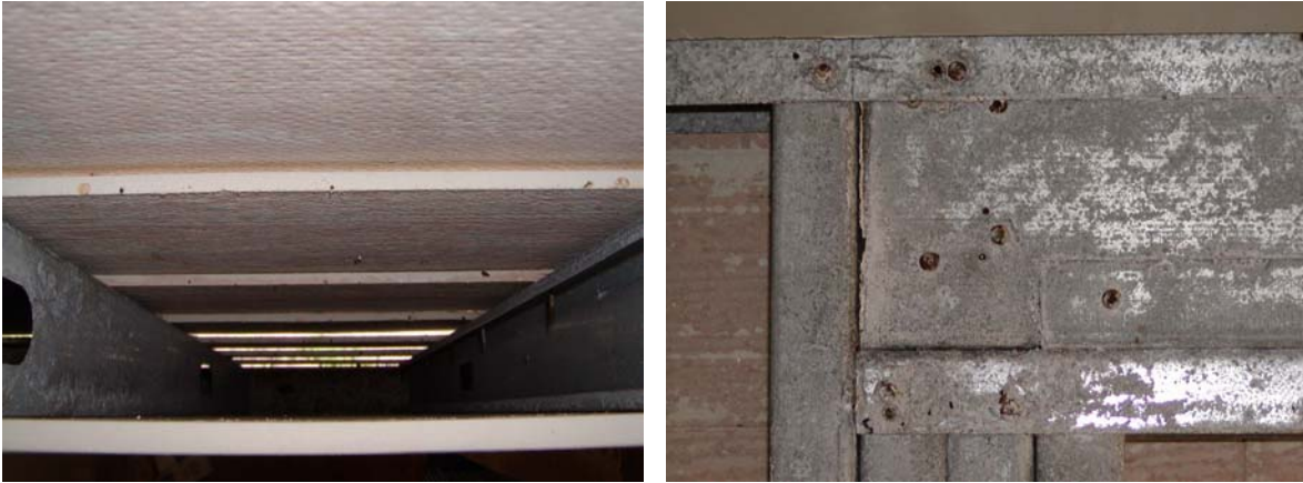
Figure 7.19: Wall framing with lap siding without vapor barrier, MCBH Coastal after 16 months.
