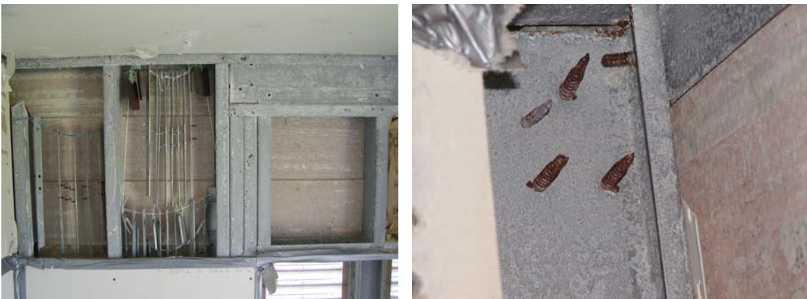
Figure 7.21: Wall framing with lap siding without vapor barrier, MCBH Coastal after 28 months.
