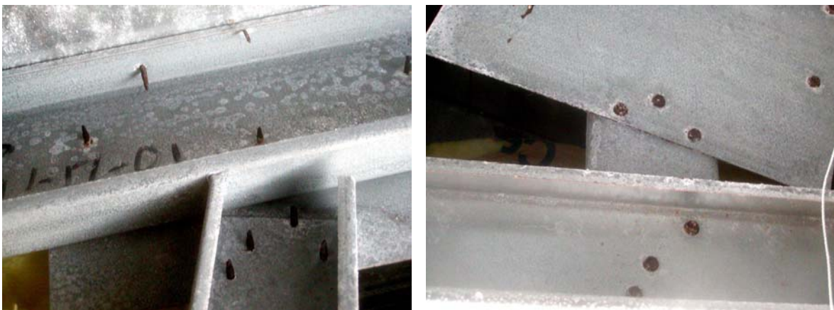
Figure 7.26: Vented attic framing at MCBH Coastal after 21 months.
