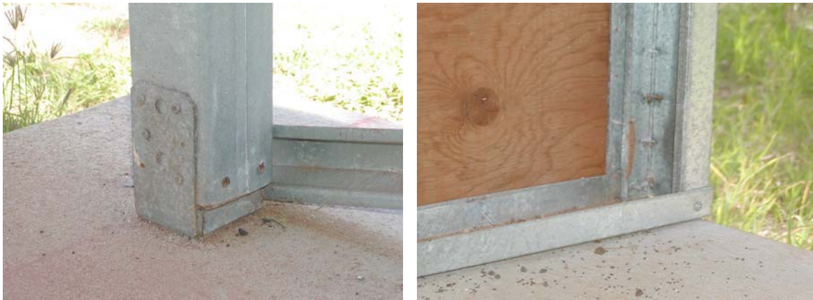
Figure 7.4: Crawl space post and cripple wall framing at Iroquois Coastal after 20 months.
