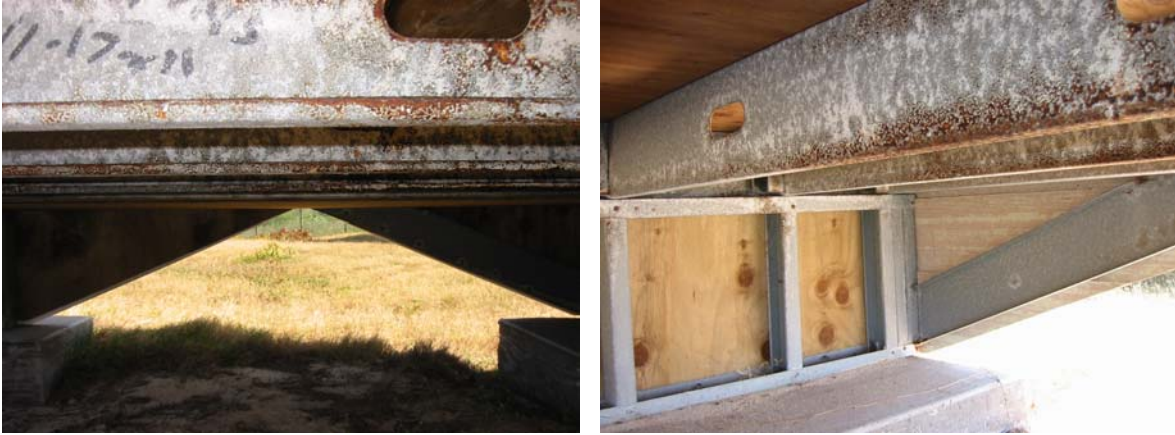
Figure 7.33: Crawl space exposed floor joists, MCBH Coastal after 10 months.
