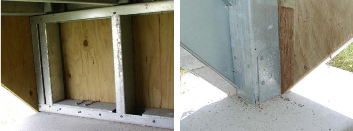
Figure 7.10: Crawl space cripple wall and post at MCBH Inland after 5 months exposure.
