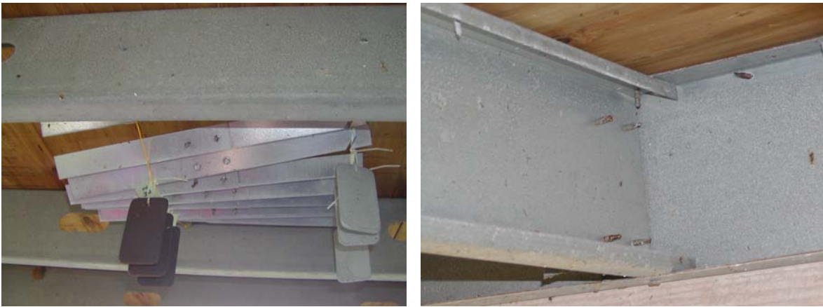
Figure 7.14: Crawl space floor joists at MCBH Inland after 28 months exposure.
