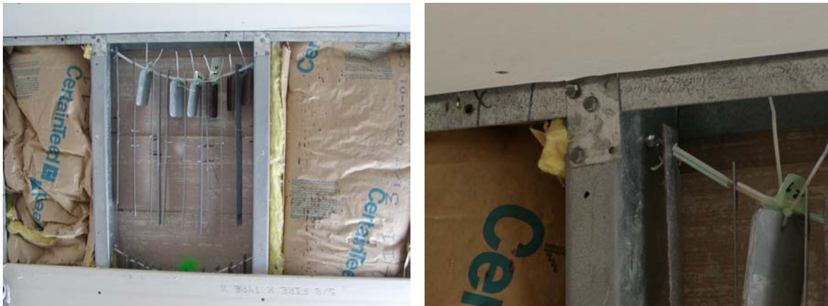
Figure 7.7: Wall framing without vapor barrier at MCBH Inland after 28 months.
