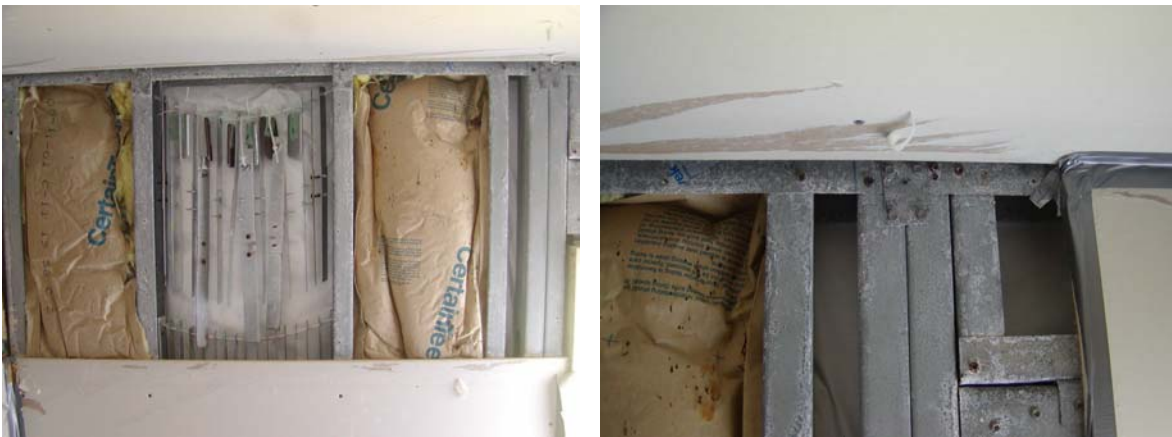
Figure 7.18: Wall framing with lap siding and vapor barrier, MCBH Coastal after 28 months.
