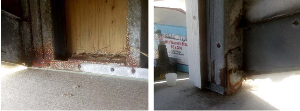
Figure 7.30: Crawl space cripple wall and post, MCBH Coastal after 21 months.
