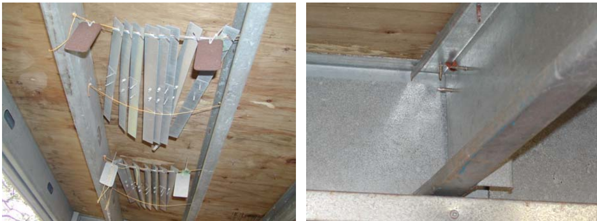
Figure 7.5: Exposed floor joists at Iroquois Coastal after 20 months exposure.
