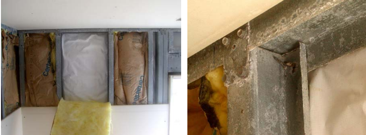
Figure 7.17: Wall framing with lap siding and vapor barrier, MCBH Coastal after 21 months.
