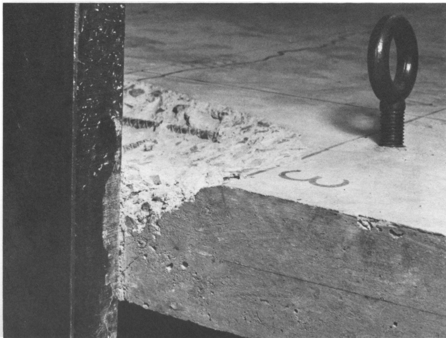
Fig. 38b B-44: End View of Failure Surface
