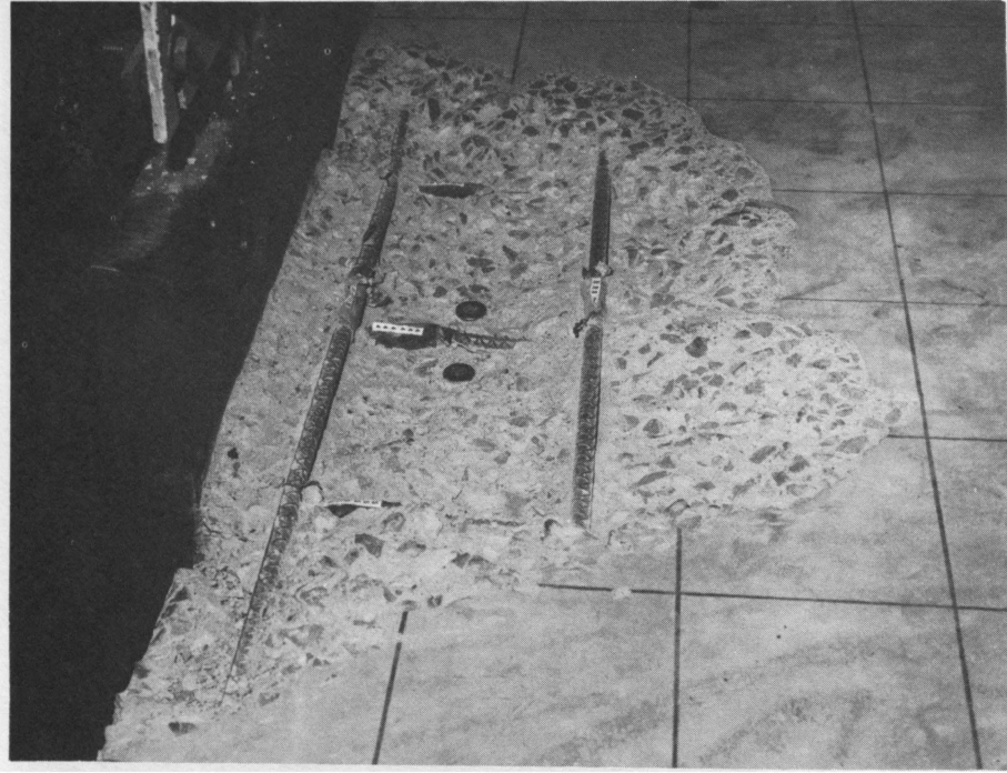
Fig. 41a B-66: Failure Surface
