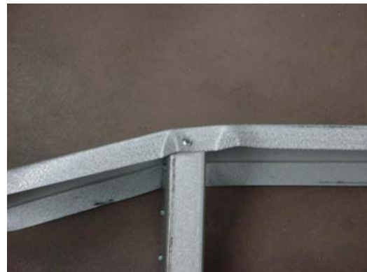
Figure 4.12-Failure of 18-ga. track
