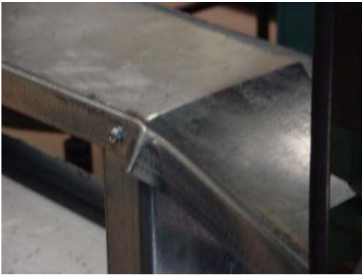
Figure 4.11-Buckling at Central Support
