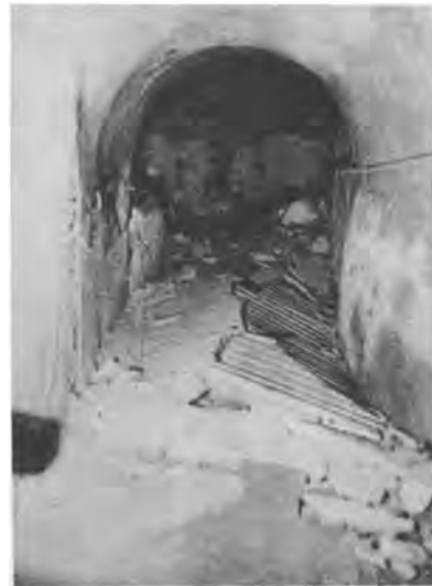
Fig.4. The most severely damaged tunnel underneath the area of I_0 = 11 . Actually the only damage was the crack of a thin concrete pavement due to lateral squeezing.
