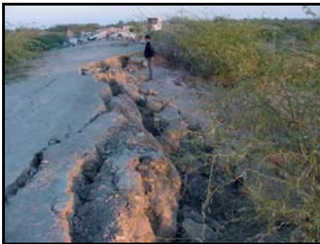
Figure 1d: Upstream slope failure of Fategarh Dam
