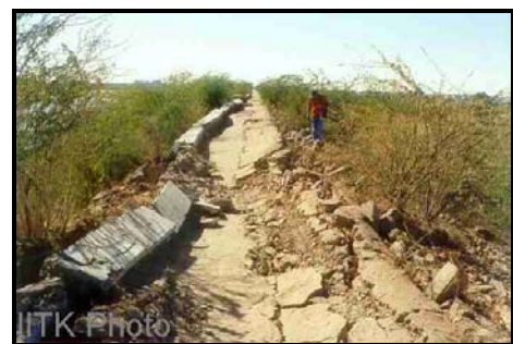
Figure 1a: Vertical and Crest settlement of Suvi Dam
