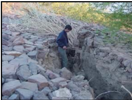
Figure 1e: Massive cracks in the upstream embankment near the toe of the Fatehgarh dam
