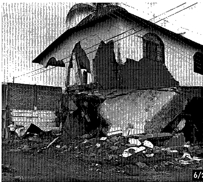
Fig. 3: Damaged modern reinforced concrete structure in Acatlán de Osorio.
