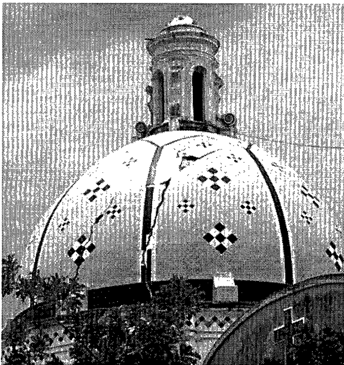
Fig. 4 : Cracked church dome in Acatlán de Osorio, typical of observed damage in the churches in the State of Puebla.
