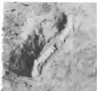
Fig.1.6 Dislocation of Buried Sewerage Pipe
