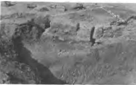
Fig.1.4 Dislocation of Wall Footing of a single storey Classroom
