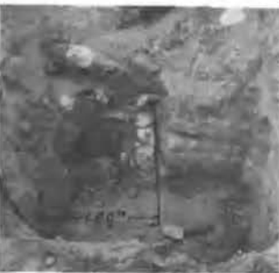
Fig.1.5 Dislocation of Brick Subway
