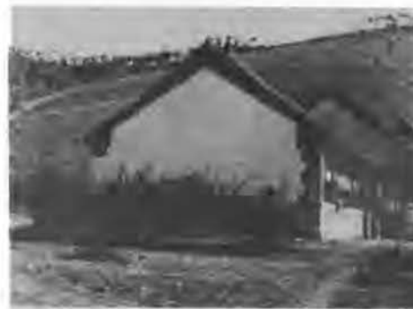
Fig.4.4 Houses nearby surface faulting (tectonic rupture about hundred meters apart) in Liao Ning earthquake stands still
