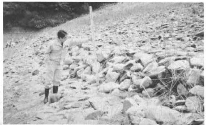
Fig. 7 Bulging on the Upstream Slope of Niwa-Ikumine Dam
