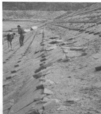
Fig. 4 Raised Facing Concrete Blocks on the Upstream Slope Protection of Mombetsu Dam
