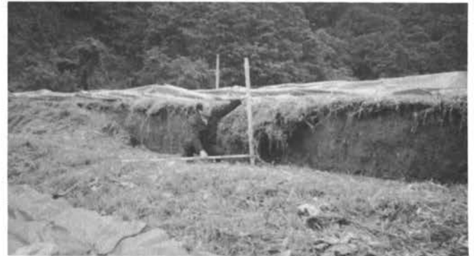
Fig. 6 Settlement of the Upstream Side Body of Niwa-Ikumine Dam
