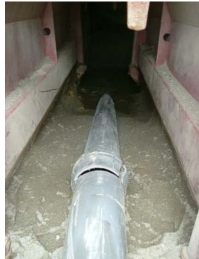
Photo 2. Uplifted pipe found during restoration work in Nagaoka City
