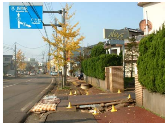
Photo 3. Road cave-in on sewage pipes in Nagaoka City
