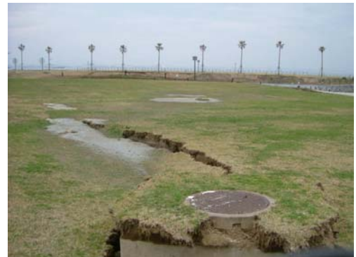
Photo 11. Liquefaction-induced flow at Uminonakamichi Seaside Park
