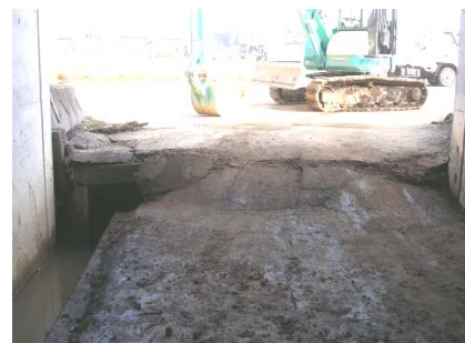
Photo 6. Settlement of culvert at C-Box Kawaguchi 22
