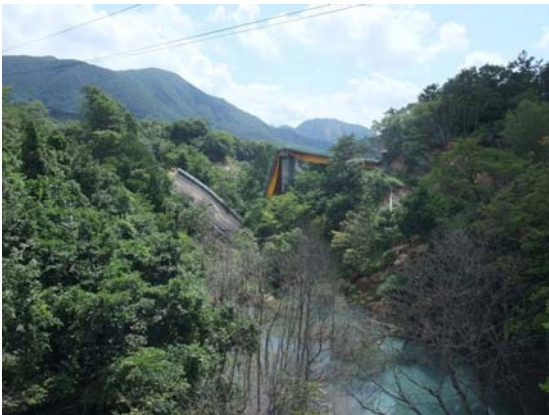
Photo 22. Collapse of Maturube Bridge
