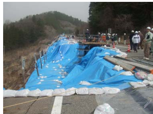
Photo 12. Slide of the embankment of Noto-yuryo road at site No.9
