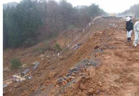
Photo 13. Slide of the embankment of Noto-yuryo road at site No.32
