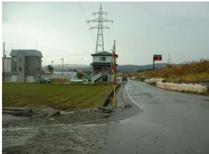
Photo 8. Moved ground adjacent to C-Box Ojiya 2
