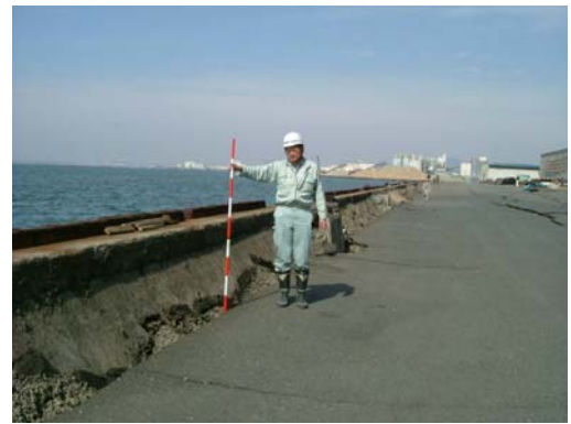
Photo 9. Displacement of a quay wall and subsidence of the ground in Oki-hama
