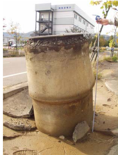
Photo 1. Uplifted manhole in Ojiya City
