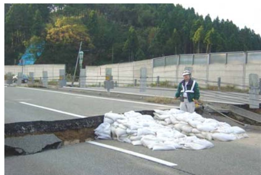
Photo 4. Differential settlement between embankment and culvert at C-Box Kawaguchi 11 (Yasuda and Fujioka, 2009)
