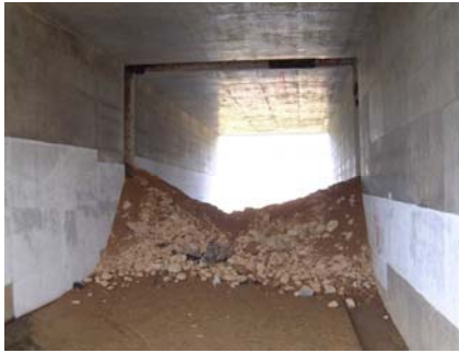
Photo 7. Separation of culvert joint at C-Box Ojiya 2 (Yasuda and Fujioka, 2009)
