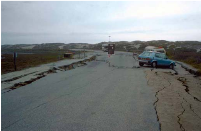
Fig. 1. Ground failure due to liquefaction during Loma Prieta earthquake 1989 ( http://earthquake.usgs.gov/bytopic/photos.html ).
