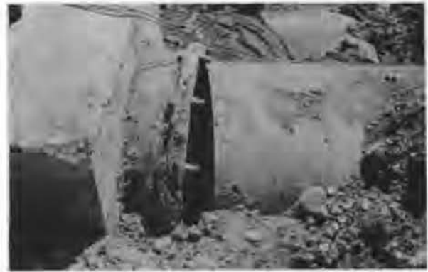
Fig. 5. Damage of Makomanai pipeline.
