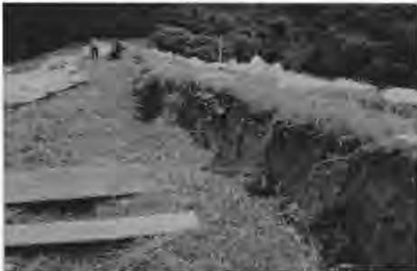
Fig. 8. Damage of Niwa-Ikumine Dam.
