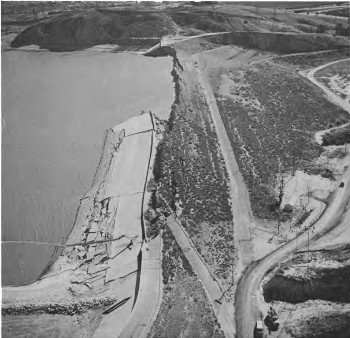
Fig. 1. View of Lower San Fernando Dam after Upstream Slope Slide in Earthquake of Feb. 9, 1971
