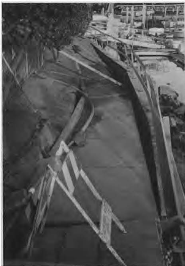
Fig. 6 Movement of the retaining wall of the pier in Redondo Beach.
