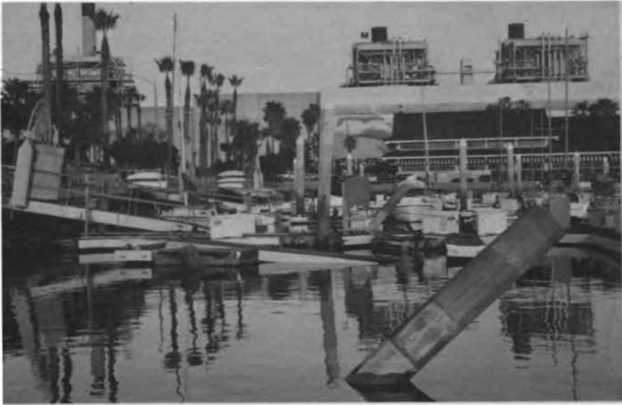
Fig. 7 Tilting of the mooring piles at the toe of the rock berm of the pier in Redondo Beach.
