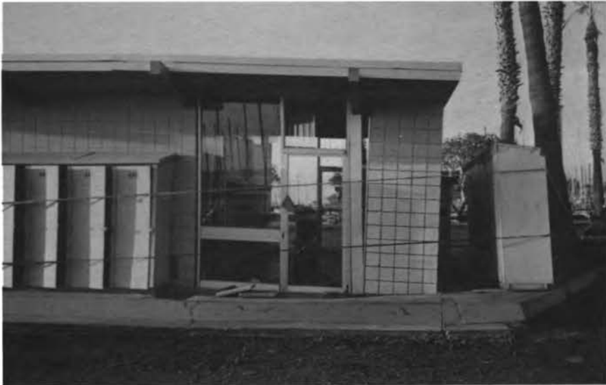
Fig. 8 Liquefaction-induced settlement of a building on the pier in Redondo Beach.
