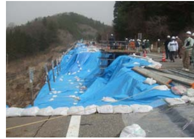
Photo. 1. Slide of the embankment of Noto-yuryo road at site No. 9
