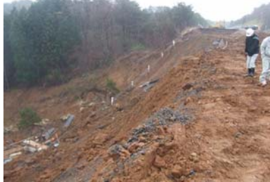
Photo. 2. Slide of the embankment of Noto-yuryo road at site No. 32
